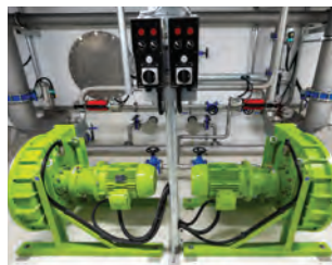
ALH65 wastewater treatment
