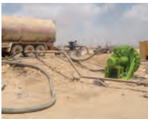
ALH125 crude oil pumping
